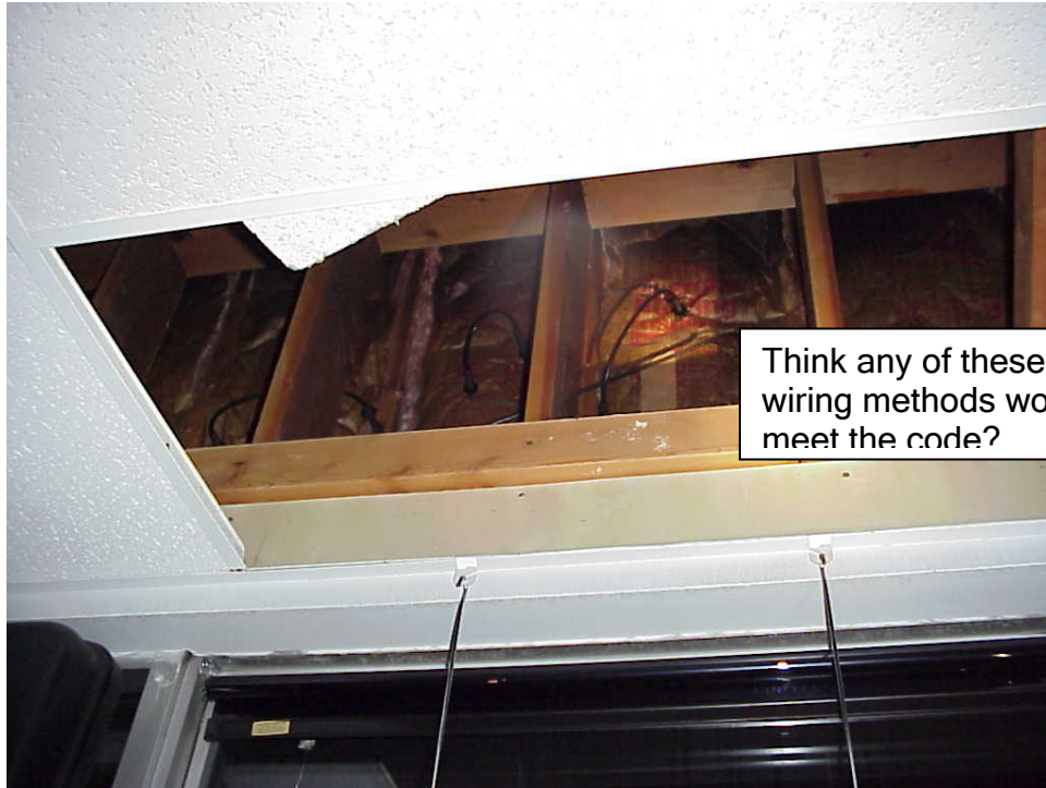
Wiring behind the wall on a set of neon channel letters.
